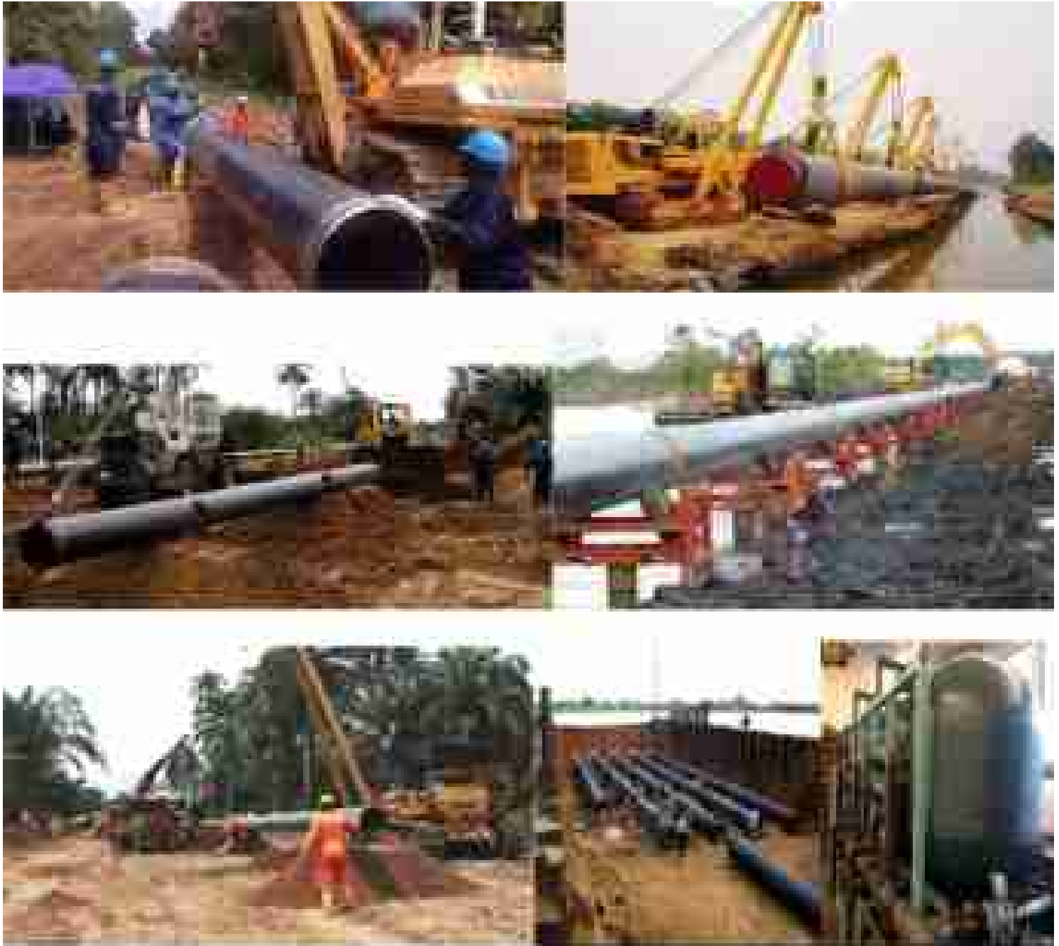
Laying of 24" Gas piping by E-18 in Nigeria Petroleum Development Company Delta State 6 Feb. 2018 to 31 Serpt. 2018 Project Contract Value: N250,000,000.00
